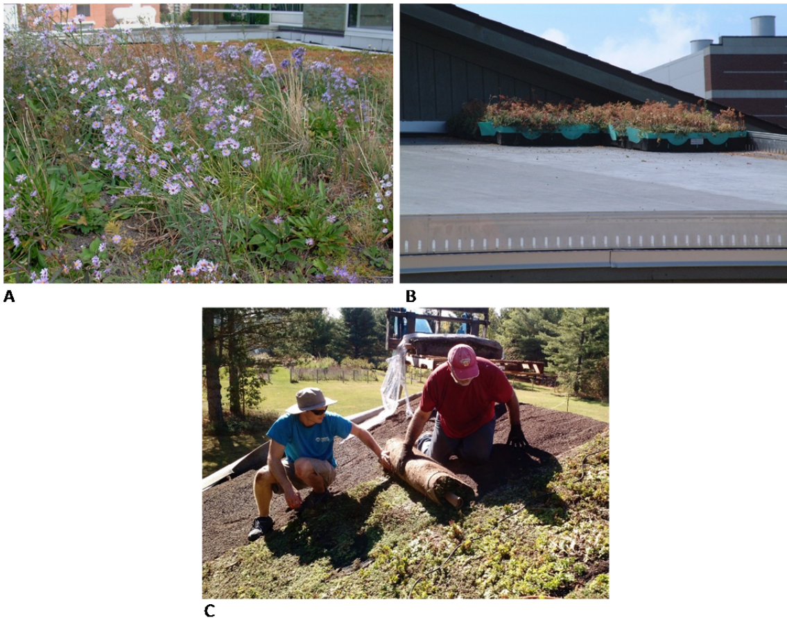
Figure 2. A. Conventional built-up green roof on the Molecular Plant Sciences Bldg. at Michigan State University in East Lansing, Michigan. B. Module green roof being installed on the 4H Children’s Garden outdoor classroom at Michigan State University in East Lansing, Michigan. C. Pre-vegetated mats being installed on a private residence in Mason, Michigan.
