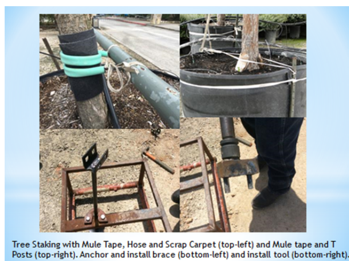
Figure 7. Tree staking with mule tape, hose, scrap carpet and mobile home anchors.
